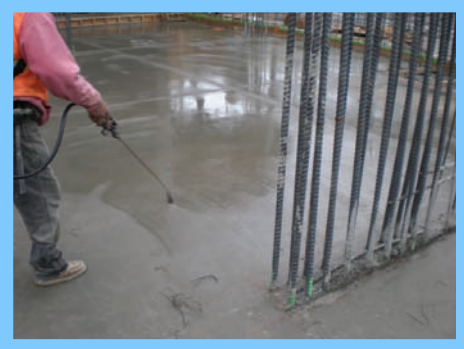
VC5™ application to cure freshly placed concrete slab scheduled for VCT and rubber-backed carpet.
