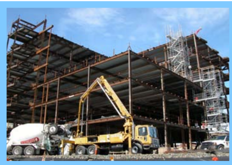
VC5™ was used to cure a 59,479 square meter hospital project sceduled to recieve moisture sensitive flooring.
